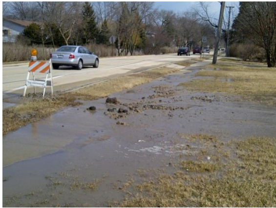
Walters Avenue Water Main Break
