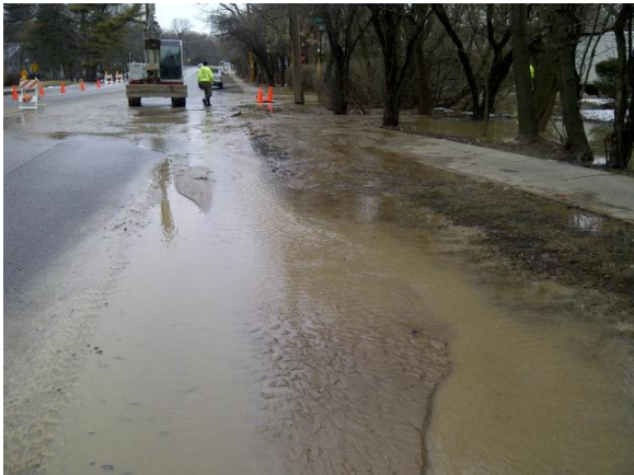
Waukegan Road Water Main Break
