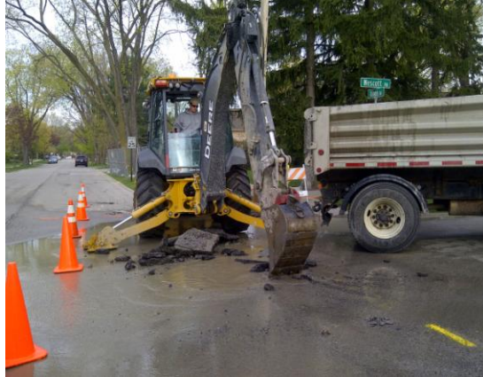
Illinois/Wescott Water Main Break
