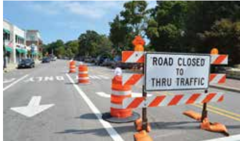
Businesses are open and there is ample on-street parking along Shermer Road during the bridge construction.
