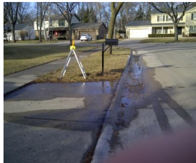
Crestwood Dr. Water Main Break
