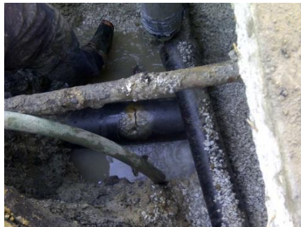
Meadow Rd. Water Main Break
