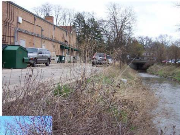
Curb Failure Looking Westerly
