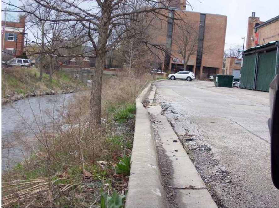
Curb Failure Looking Easterly
